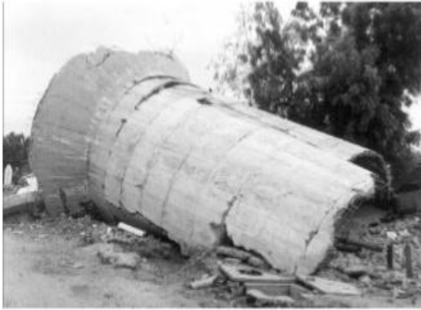
Figure 1: Collapse of water tank in Bhuj
