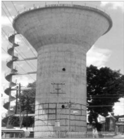
Figure 2: Flexure cracks in staging
