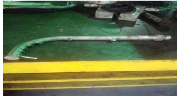
Figure:2 Banana Receiver Pipe for cooling arrangement.
